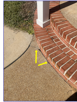
Minor cracking in walkway at front porch step area. Recommend sealing area that is cracked to help prevent future damage.
