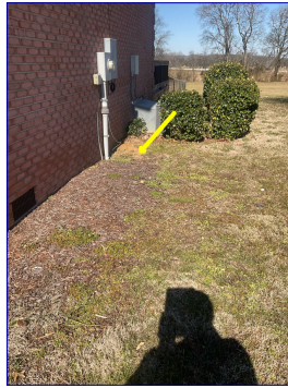
Water is ponding at foundation located by electrical meter base. Recommend additional backfill so water will drain properly from foundation.
