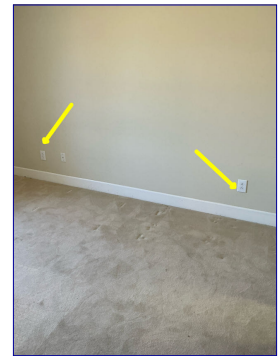
There are several loose receptacles in the northeast guest bedroom. Recommend electrician make necessary repairs.
