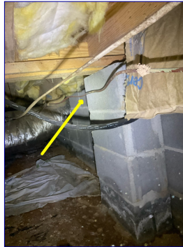
Copper gas line in the crawlspace will need to be secured floor joists if gas is installed.
