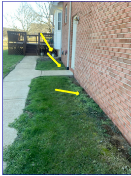
There is a negative grading slope, toward the foundation, in one or more locations. Recommend maintaining a positive drainage slope away from the foundation. Consult a professional landscaper for proper drainage and grading as needed.
