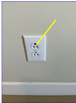
Loose and broken receptacle in northeast guest bedroom. Recommend electrician replace receptacle.
