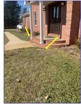
Water is ponding at each side of front porch area steps. Recommend additional backfill be added.
