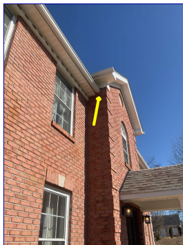
Gutter attachment above front porch area located at West side of porch area will need to be secured. Gutter is not pitched properly.
