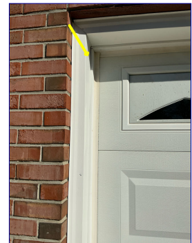
Loose trim at outside garage overhead door. Recommend contractor make necessary repairs.
