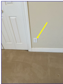
Loose receptacle on the east wall of the north west guest bedroom. Recommend electrician make necessary repairs.
