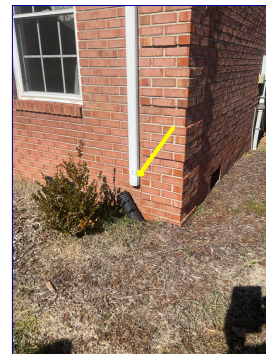
Gutter downspout at Southeast corner of house is not directing water away from the foundation. Recommend attaching back to black flex drain pipe.
