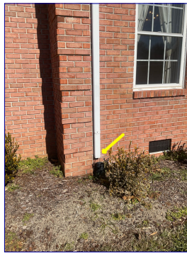
Gutter downspout at south side of house is not discharging water away from foundation properly. Recommend downspout be extended to flex drainage pipe.
