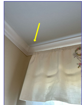
Moisture stain on the ceiling of the north west guest bedroom. No moisture was detected at time of inspection. Recommend monitoring and repairing as needed.
