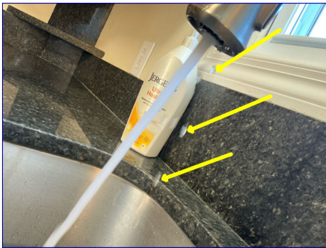
Dripping in areas of kitchen faucet when operating. Recommend plumber make necessary repairs.
