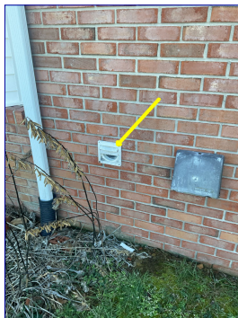
Dryer exterior vent hood will need to be replaced.
