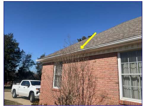
Gutter attachment at Southside of garage area will need to be re-secured and also drip edge flashing will need to be reinstalled and secured under shingles.
