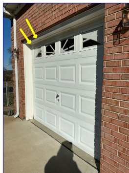
Area of wavy trim at garage door. Recommend contractor make necessary repairs.
