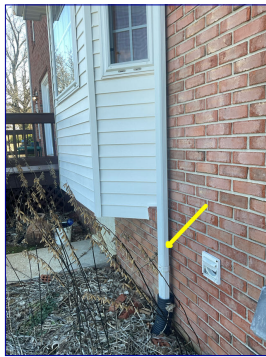
Gutter downspout beside dryer vent hood needs to be secured to siding.
