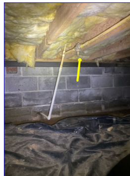
Water pressure regulator is located in the crawlspace at South wall
